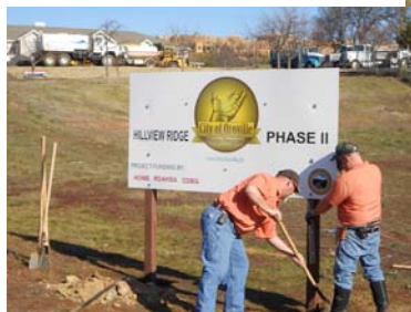
Public Works staff Jeremy Wachtel and Ron Dodd placing a MIDAS sign at the Hillview Ridge project
